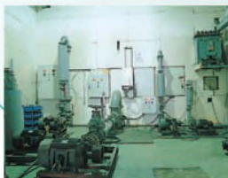
Testing area for Roots Blower
